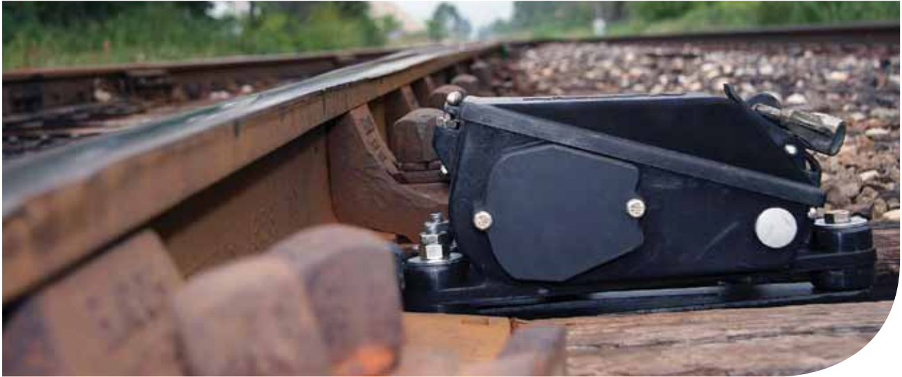
7R Switch Circuit Controller in service at customer location
