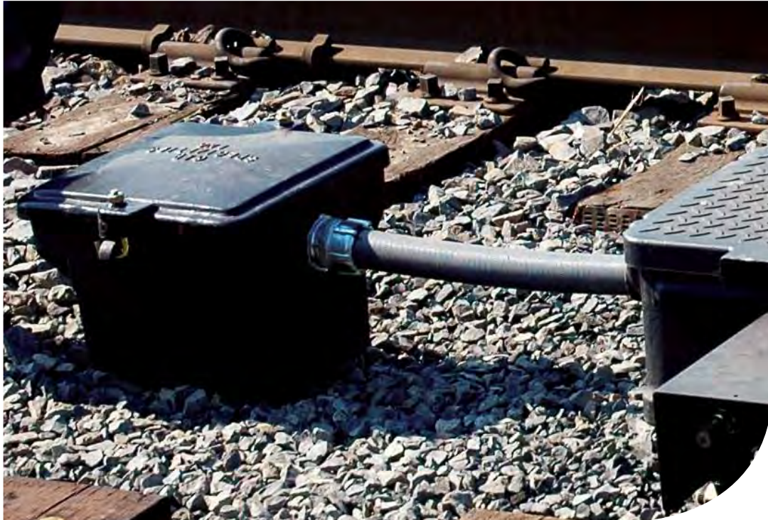
Junction Terminal Box installed at customer location
